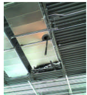
HVAC installer solution to a sprinkler installation interference
