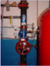
Sprinkler riser with foam tank
